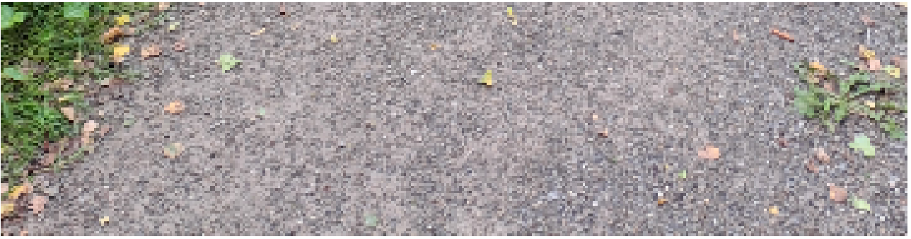
Vandalism damage to the wooden bridges in the Bocholt municipal forest © Stadt Bocholt
