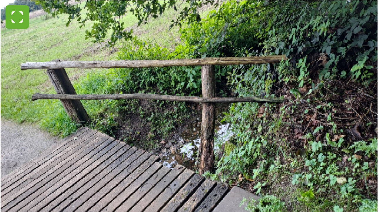
Broken wooden bridge at the Hochzeitswald in Bocholt. © Stadt Bocholt
