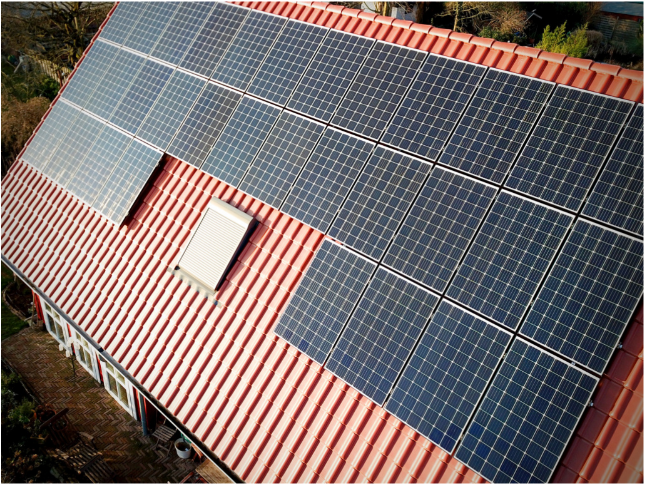
Photovoltaics or solar thermal provide electricity or heat from solar energy © Stadt Bocholt
