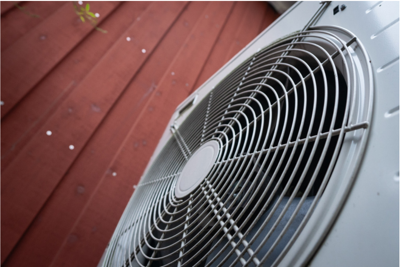
Part of an air source heat pump © Stadt Bocholt
